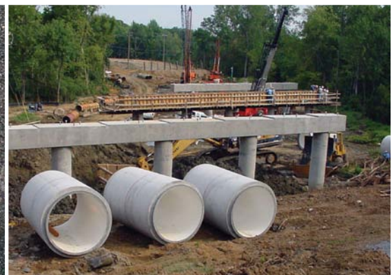
By 2020, up to half the assets in US sewer systems may be beyond the midpoint of their useful lives, which is generally assumed to be about 100 years. (Source: Optimization of Collection System Maintenance Frequencies and System Performance, a 1999 study prepared by the American Society of Civil Engineers under an EPA Cooperative Agreement)
