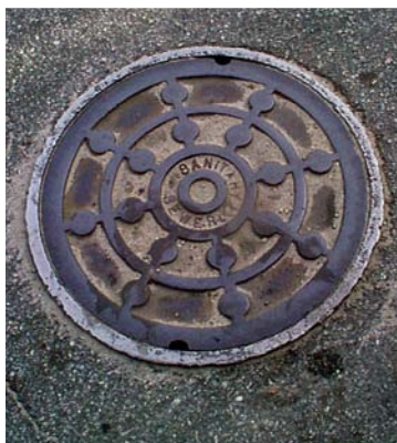
Generally, 5-10% of manholes are buried or covered by pavement.
