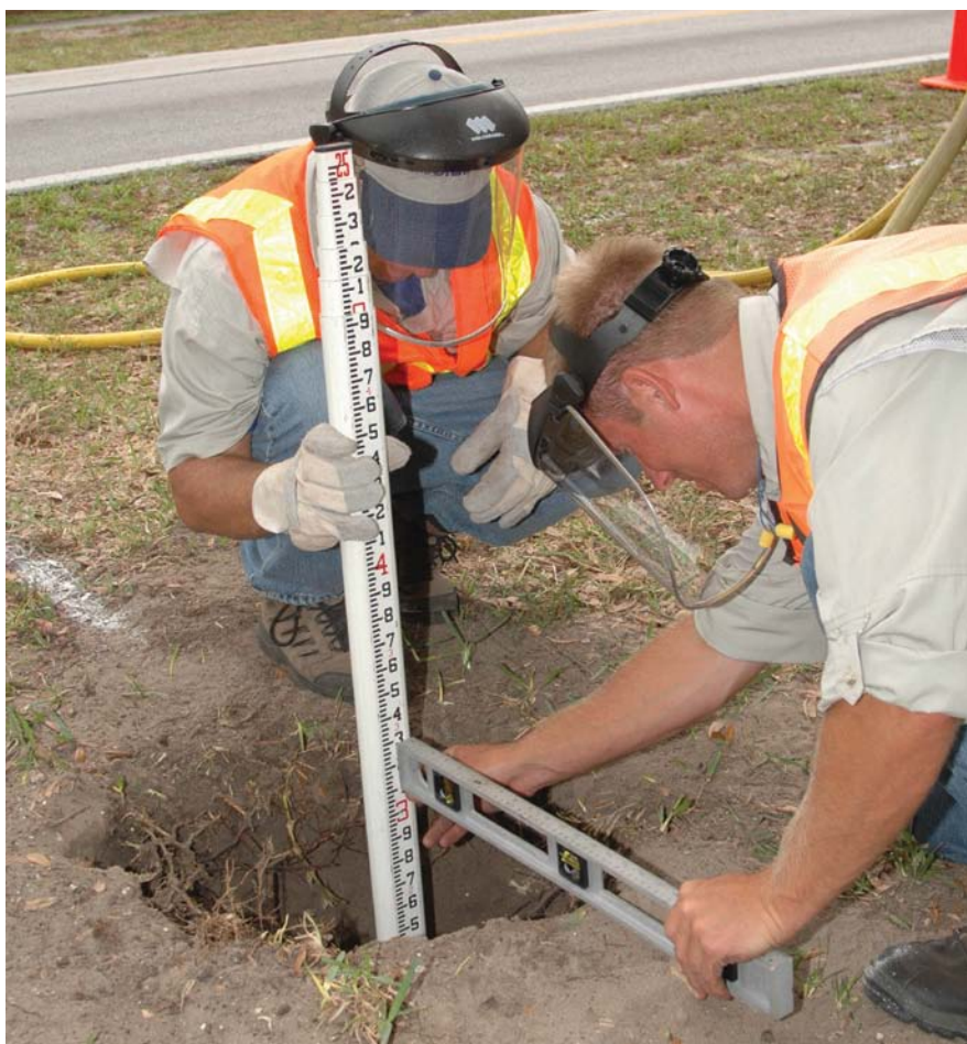
Test hole excavations enabled the team to verify horizontal designations, depth, material and size of the underground utilities along the proposed interceptor alignment.
