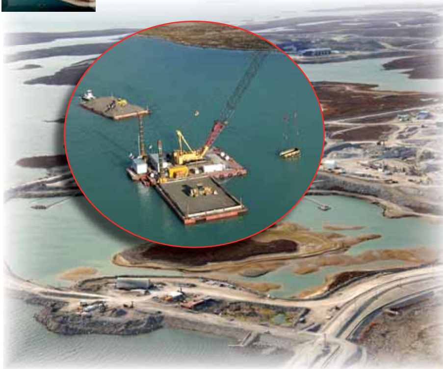
▲ In operation, the crane/barge setup (inset) has material barges flanking it and an eight-cubic-yard bucket (right) for placing gravel to form the dikes. (Image courtesy of Diavik Diamond Mines Inc.)
